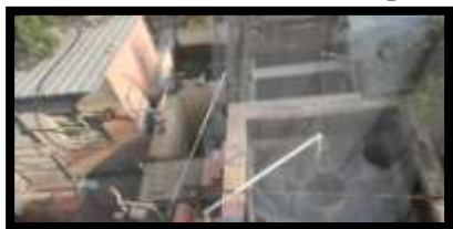
FIGURE-4 EFFLUENT TREATMENT PLANT
